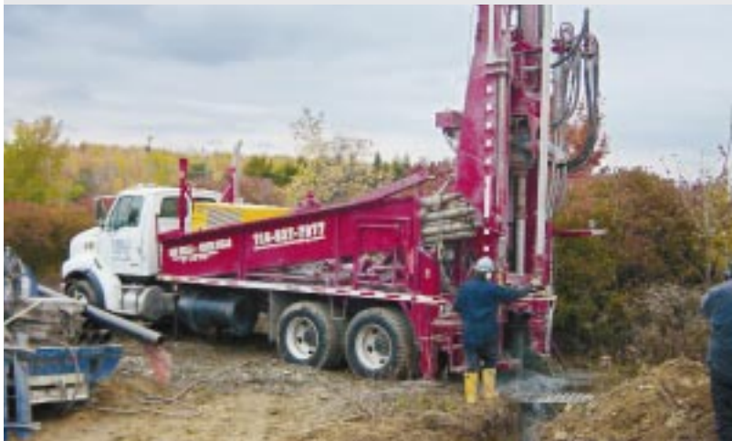
DR-12 with optional pipe tub and single rod loader in domestic waterwell application
