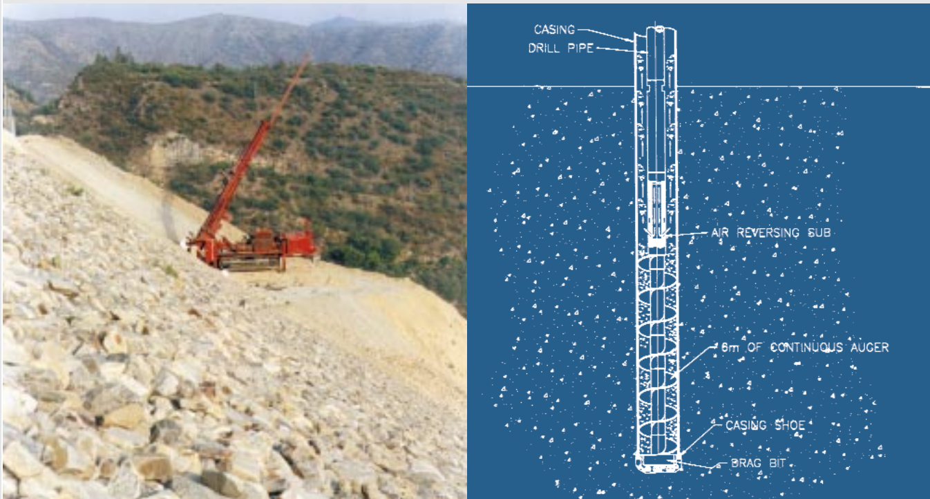
Foremost DR-24 working at dam site. Because of concern over blowout potential, an air-reversing sub was positioned 6m (18ft) above the drill bit to divert air flow back up the annulus to clear cuttings from the auger string. The tooling configuration created a low-pressure vacuum at the bit, eliminating the possibility of a blowout.
